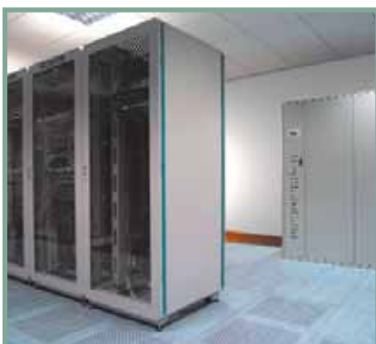
Data centre cooling
